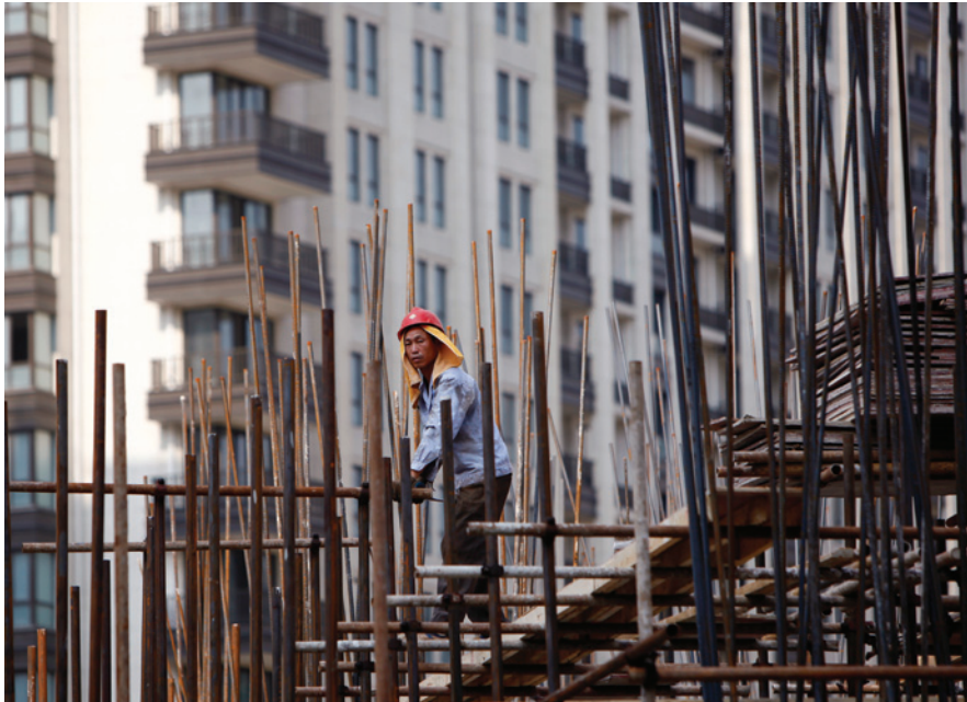
A migrant labourer works at a construction site in Shanghai August 1, 2010. REUTERS/Ally Song
