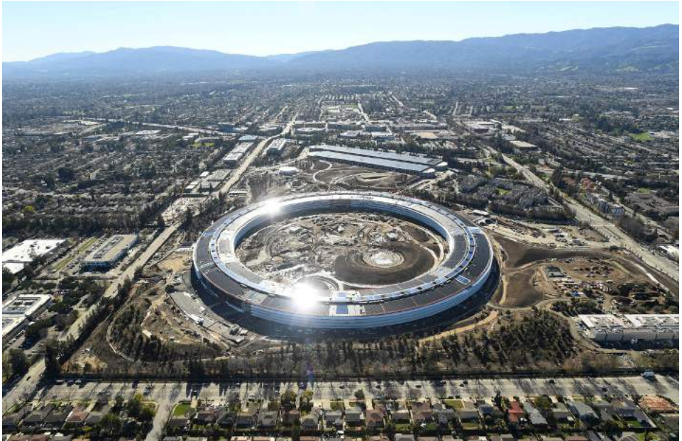
The Apple Campus 2 is seen under construction in Cupertino, California in this aerial photo taken Jan. 13, 2017. REUTERS/Noah Berger
